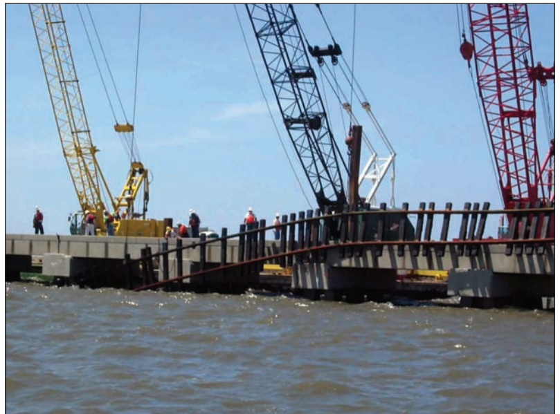
Cranes pulled rail from the lake and placed it back on the bridge surface.
