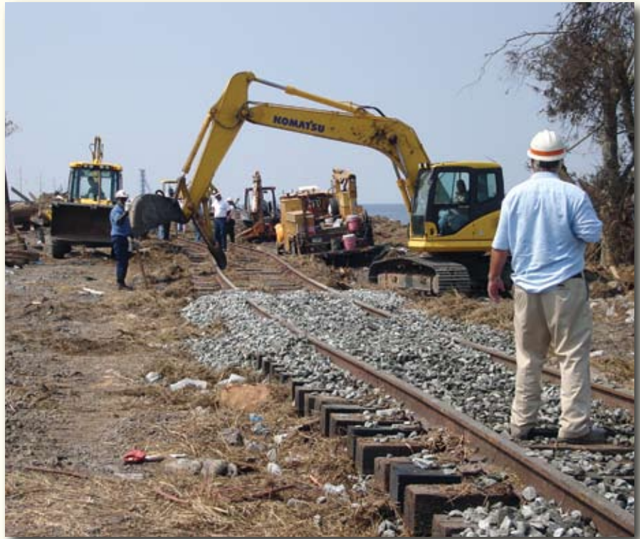
People and machinery join forces to repair a section of track damaged by Hurricane Katrina.
