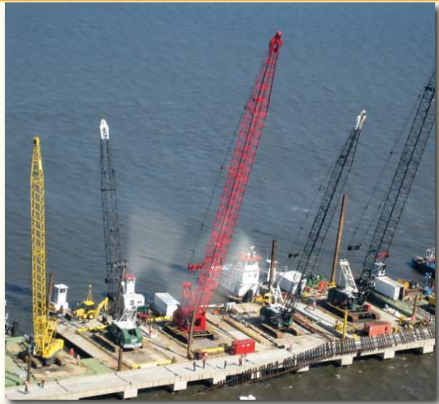
Floating cranes all in a row tower over the barren deck of the Lake Pontchartrain trestle following Hurricane Katrina. As seen at lower right, the cranes recovered 4.8 miles of track from the lake and lifted it back onto the bridge.
